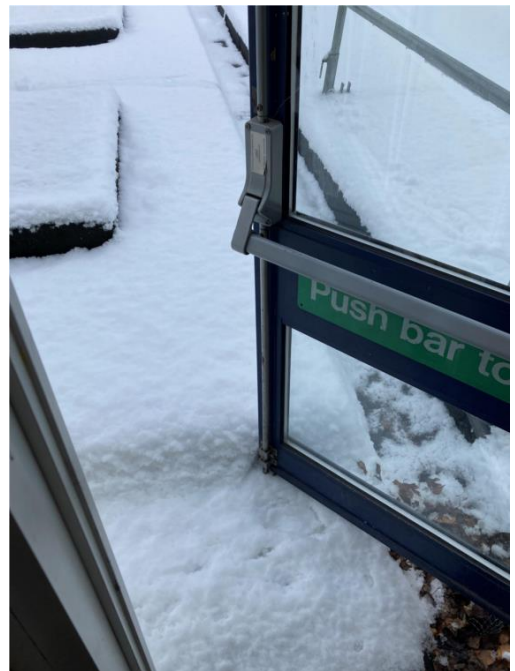
blocked escape route (partial)
