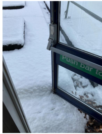
blocked escape route (partial)
