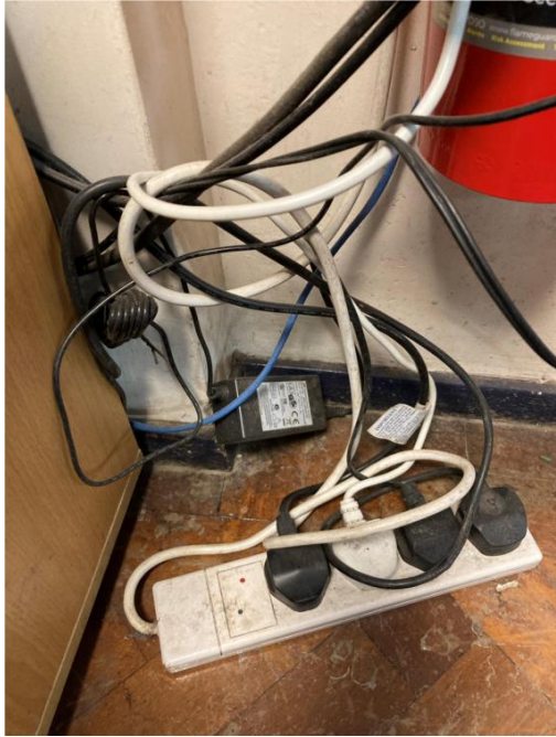
PAT testing needed throughout
